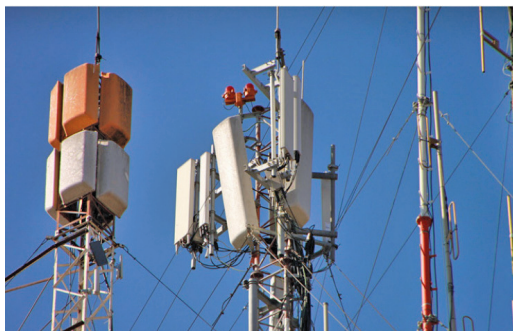
Figure 3. Base transceiver station (BTS)
